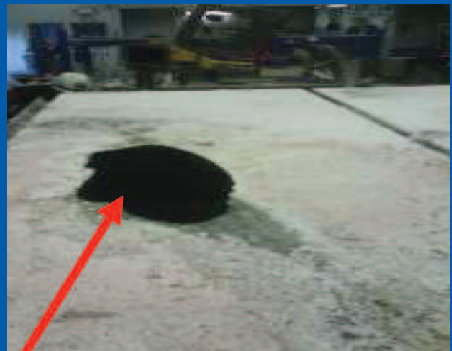
Hole is top cover due to internal arc energy
