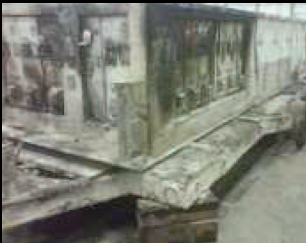
Depiction of standard underground electrical equipment after being subjected to an internal arc.
